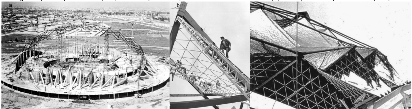
Figure 7. a) Assembly of the arches b) Sample of assembly of secondary structures over the structure of arches; b) Assembly of the deck. (Villasana Suverza, 2015).
